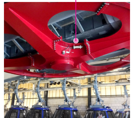
In the valley station, the deflection roller of a chairlift is lubricated with two simalube 250 ml lubricators.
