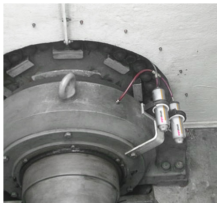
Two simalube 250ml lubricators lubricate the main bearing of a wind turbine.
