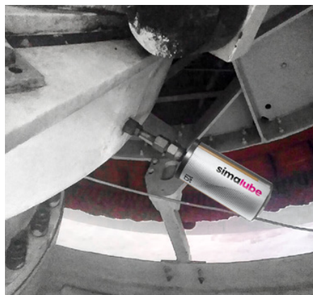
In this wind turbine, the simalube lubricator is set with a dispensing time of six months.
